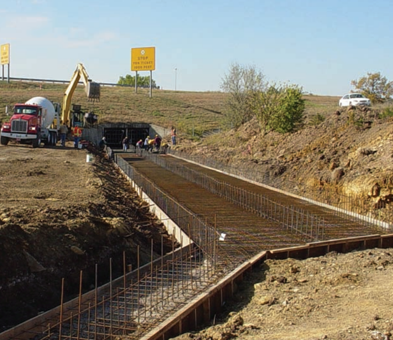
Left: Concrete work begins on the maintenance tunnel for the new Emporia plaza.
