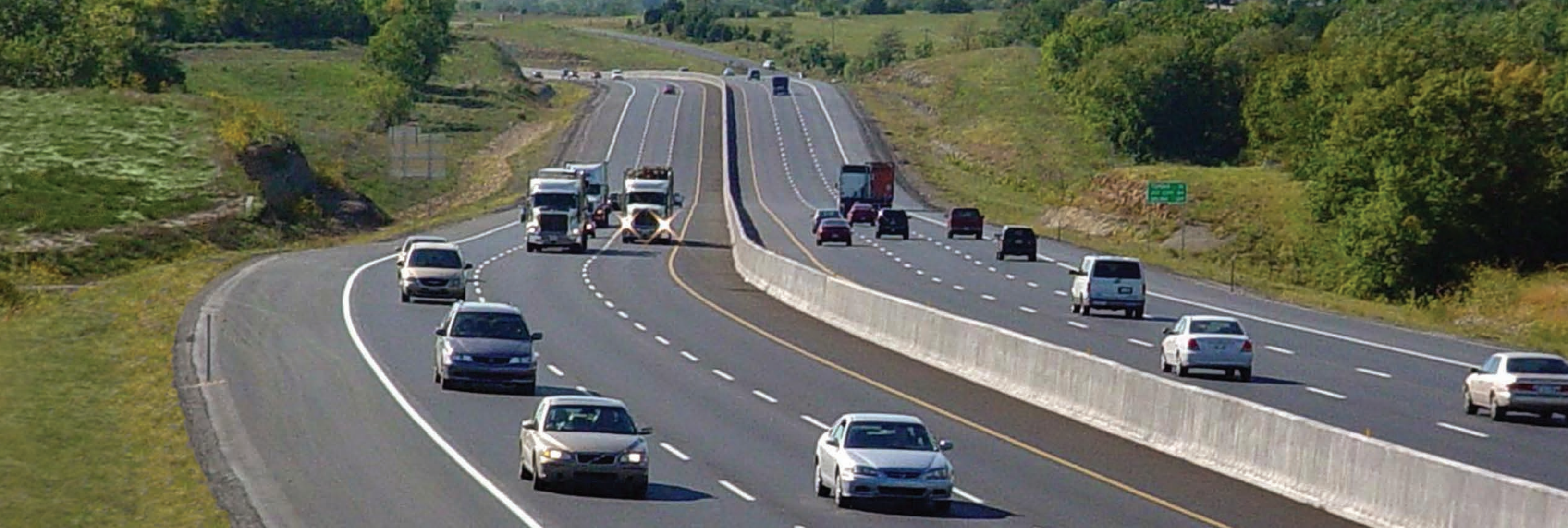
Creating a wider ride. Sections of six-lane traffic opened in the construction area in the fall of 2006. By the end of the year, work on the project was 94 percent complete while only 82 percent of the estimated construction time had passed.
