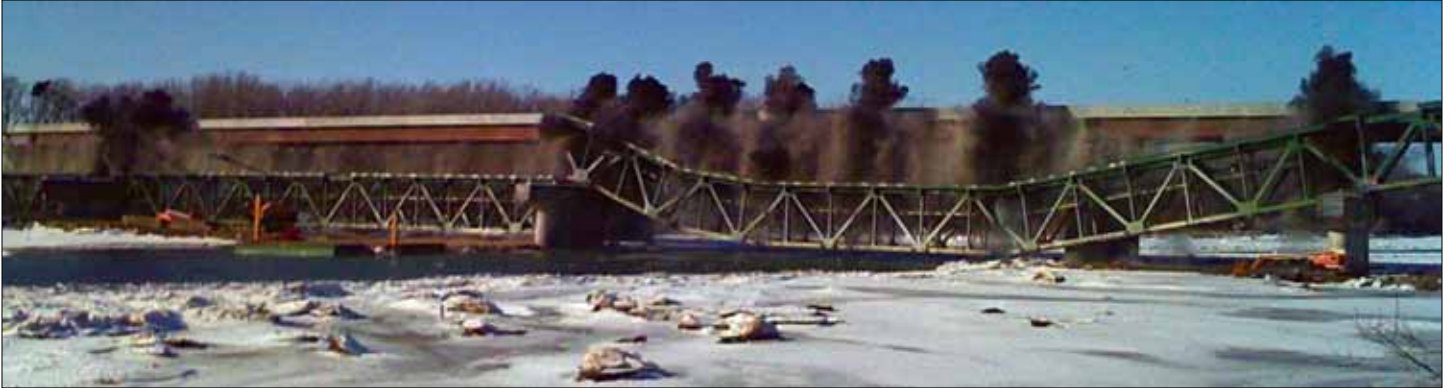
The last and largest section of the out-of-service Kansas River Bridges is dropped using explosives. The two bridges were dismantled in sections on six different dates between Nov. 15, 2009, and Jan. 13, 2010. Machines then "chewed" the large trusses up so the metal could be removed for recycling.
